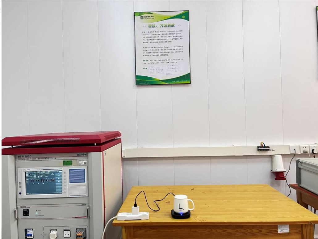
Photo of Harmonic & Flicker Measurement
