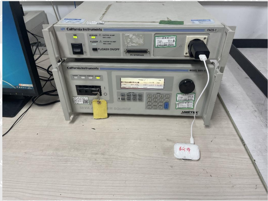
Harmonic/Flicker Test View
